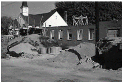
Pictured above is the building of Steinbicker Hall in 1953. Construction was completed in June of that year.
